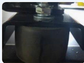
Anti-vibration mounts fitted to prevent vibration and noise.
